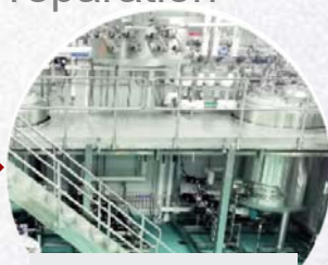
Purification system 纯化系统
