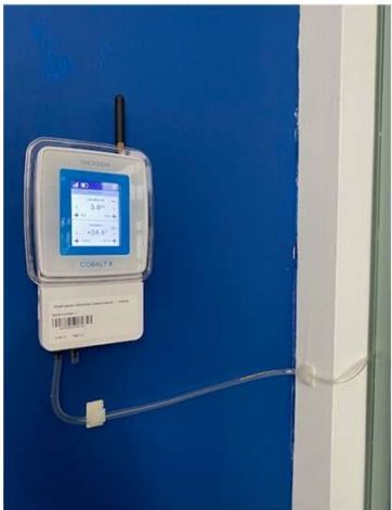
Clean room / Climatic Chambers (Cobalt X / Differential Pressure Sensor)
