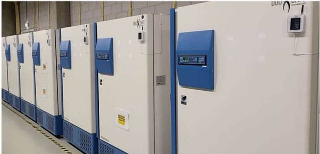
Freezers Farm (Cobalt X / PT 100 sensor)
