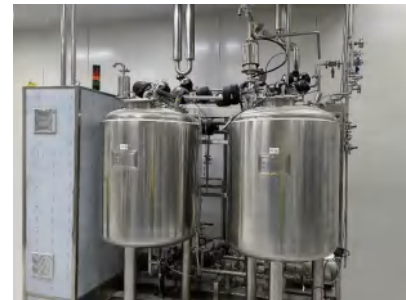
Wastewater and Exhaust gas treatment Module
